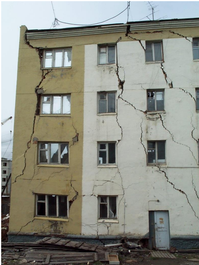
Figure 9. Residential block in Cherskiy, damaged as a result of the weakening of foundations built on permafrost. Photo: Professor Vladimir Romanovsky.
